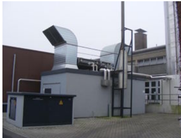
Concrete Sound Enclosure
